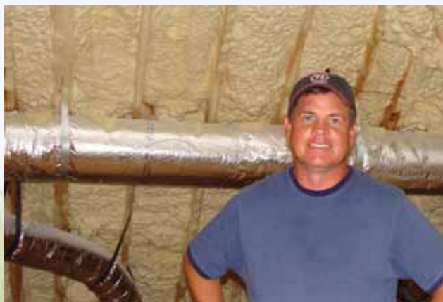
The spray foam insulation in Underwood's home expands to 120 times its volume.
