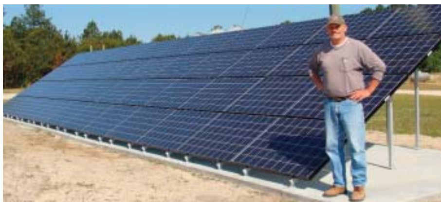
Lee Hosking is very satisfied with the installation of his 10.9 kw solar array.
