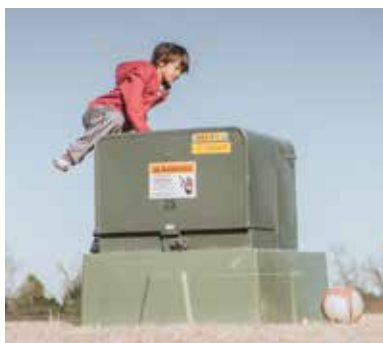
This is an electric safety hazard.
